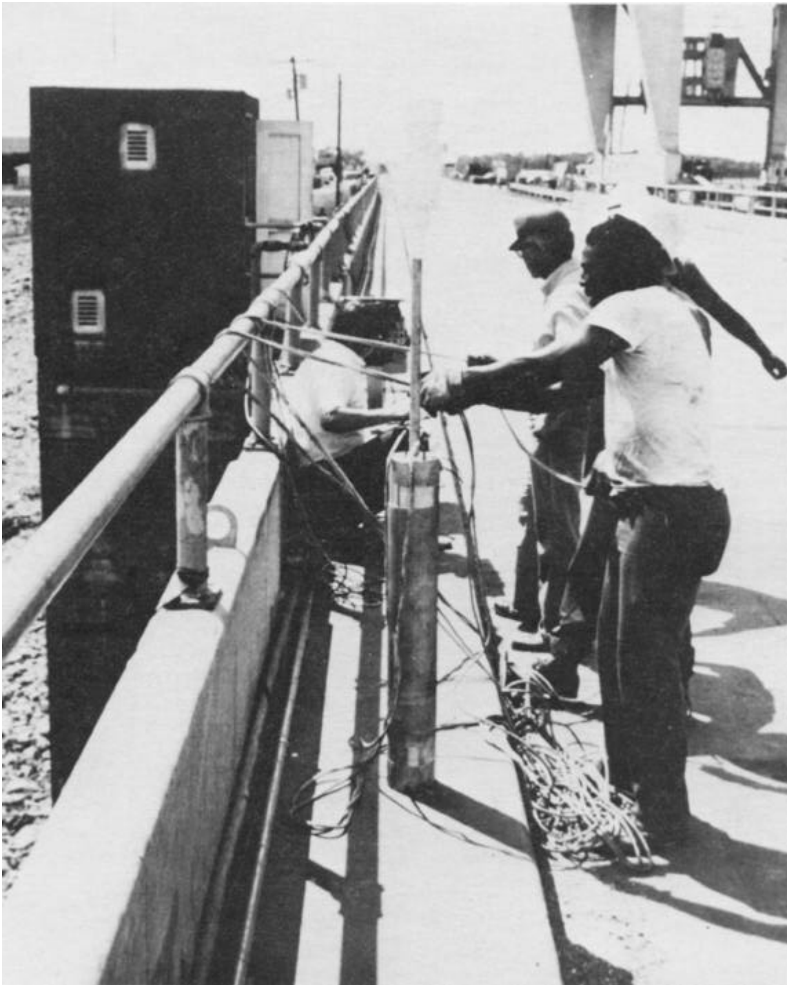
Figure 3-9. WES Pressure Measuring Telemetry System. (Photo by WES)
