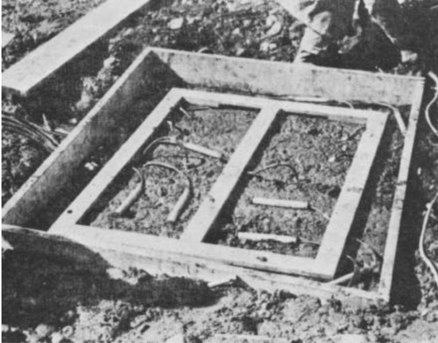
Figure C-1. Strain Meter Group Ready to be Covered (Courtesy of the Bureau of Reclamation).
